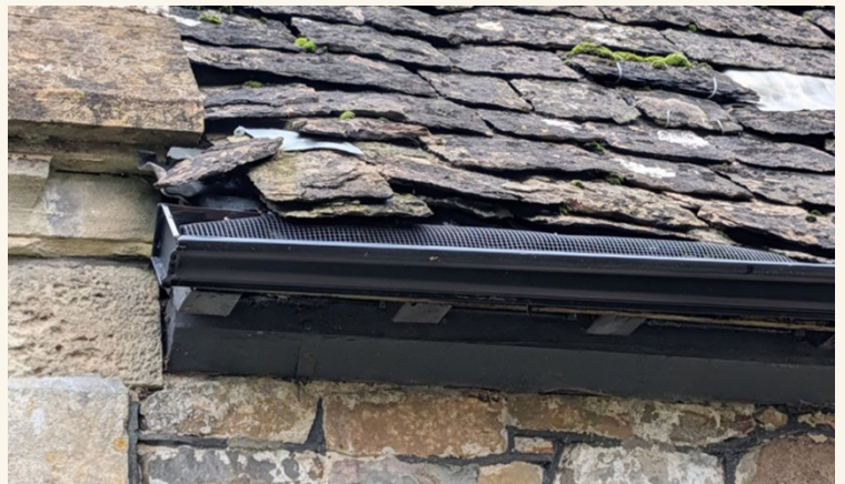
STONE SLATES DELAMINATING AFTER MORE THAN 150 YEARS OF ENGLISH WEATHER
