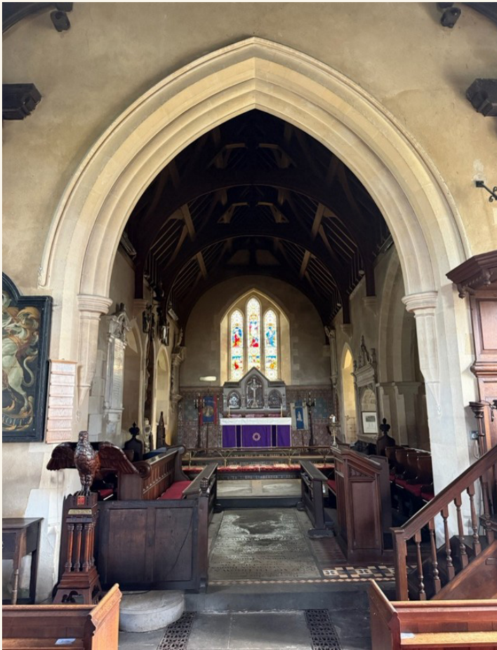
THE BEAUTIFUL CHANCEL - AT RISK IF THE ROOF FAILS
