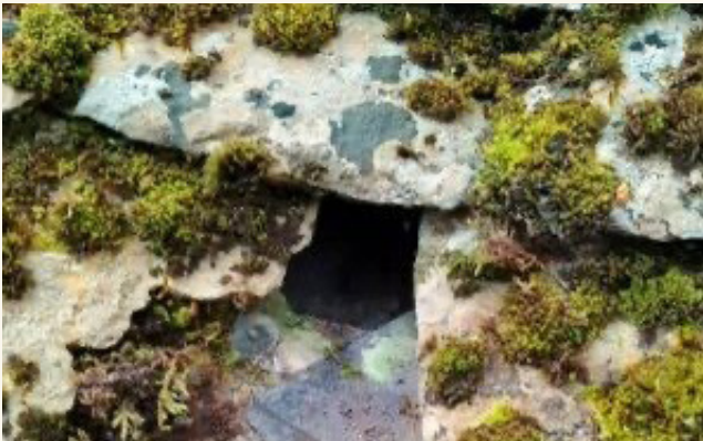
GAP IN THE ROOF - DAYLIGHT VISIBLE THROUGH FAILED SLATES
