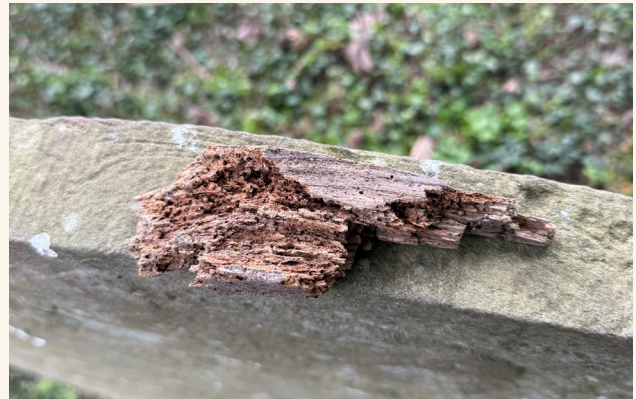
ROTTEN BATTEN CAUSING TILES TO SLIP - THE HIDDEN FAILURE BENEATH THE SURFACE
