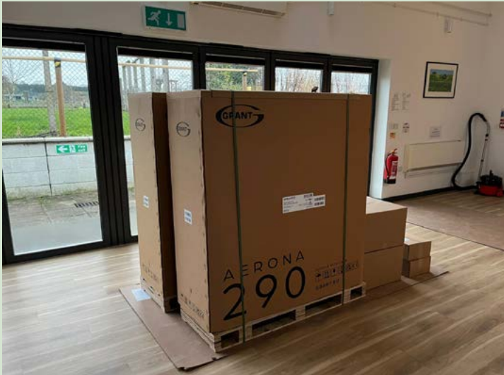
Air Source Heat Pump delivered and installed, the plant room and the piping
